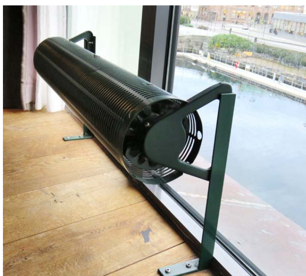
Installed by a window the ribbed pipe radiators effectively counteract cold draughts that frequently form by large glazed areas.
